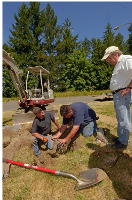
Nisqually Public Works Manager Tom Arnbrister discusses a change that needs to be made to make sure a few of the new water meters on the reservation are flush with the ground after installation. Working on the fitting are Brian Peterson and Joseph Johns II.
