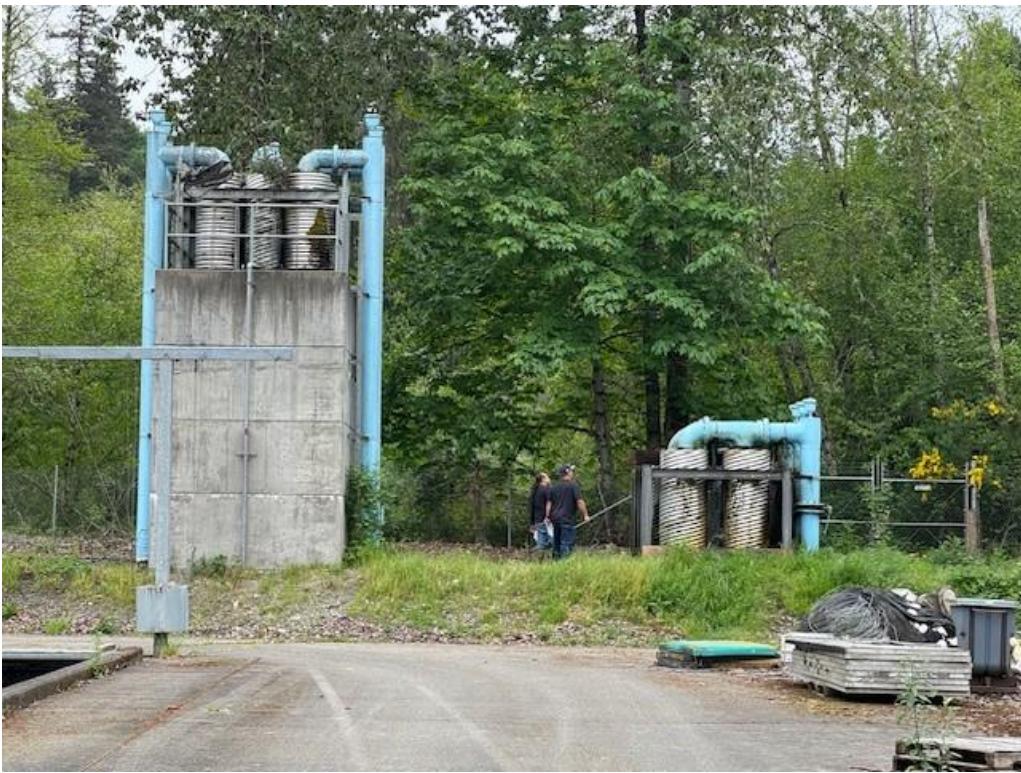
10 – Aeration Towers (men for scale)
